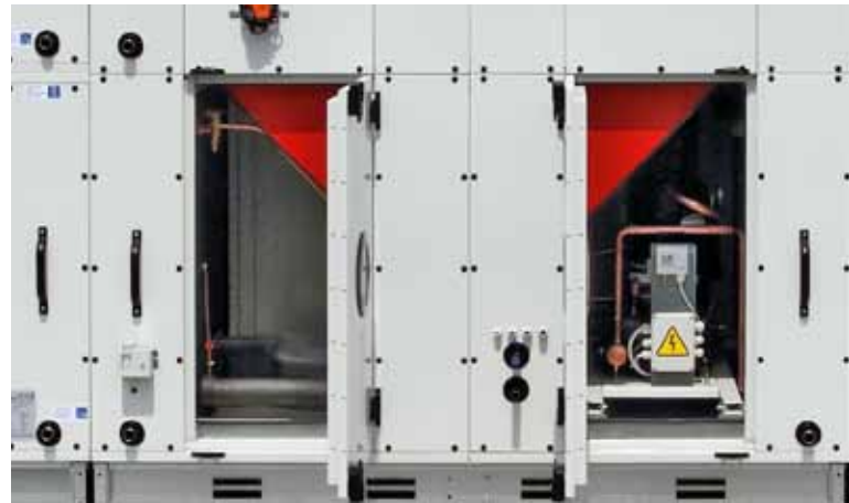
Swimming pool (Swiss) – dehumidification, ventilation and heating of the swimming-pool hall
